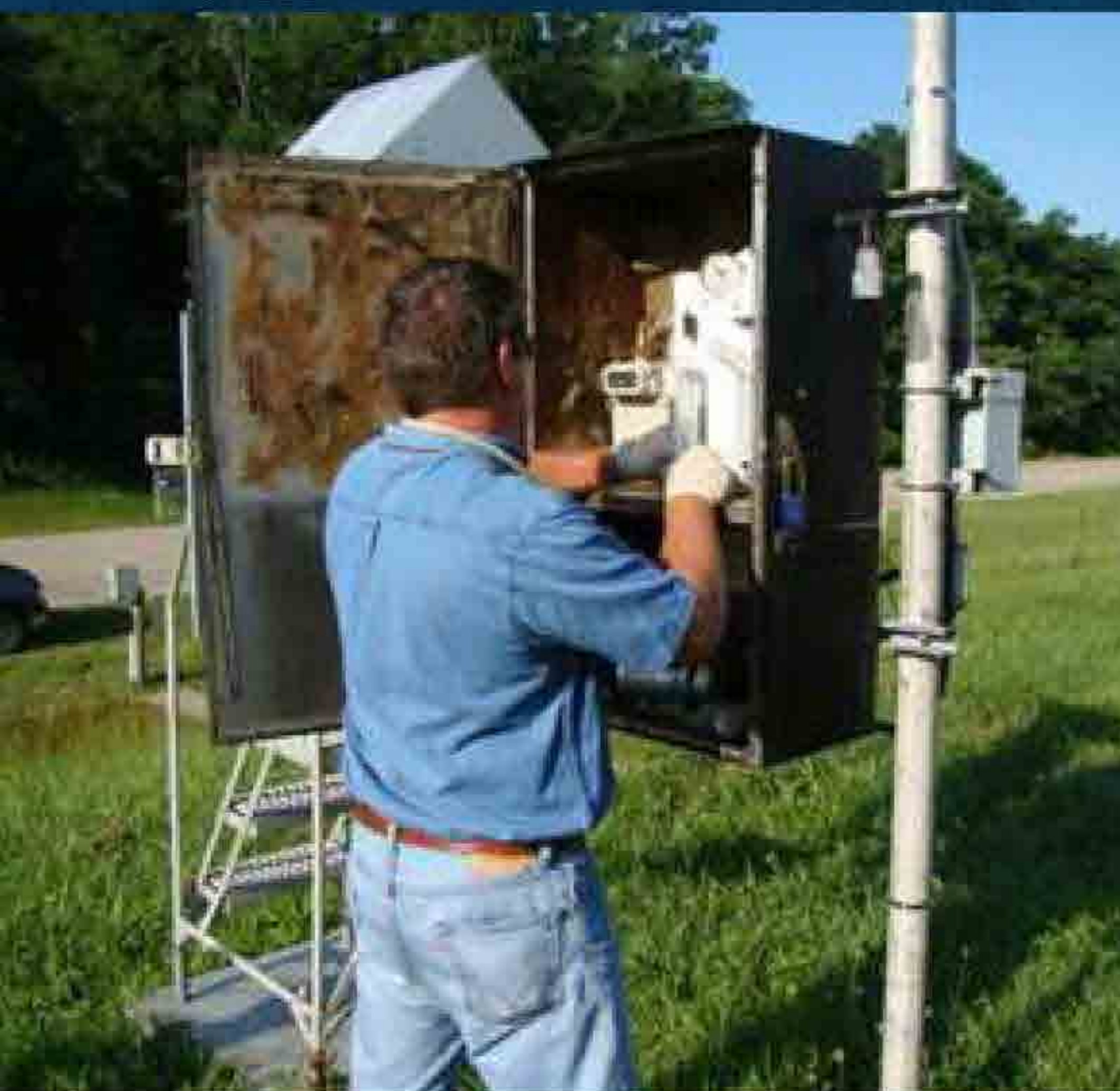
Air Monitoring Station
